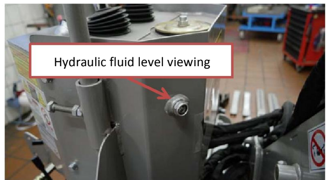
Fig.9 Hydraulic fluid level viewing glass
